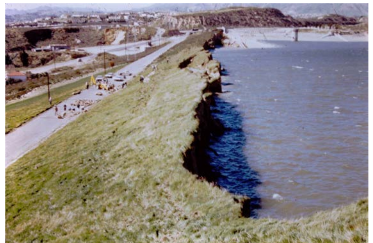
Lower San Fernando Dam – remains of crest after upstream slope failure – LADWP photo
