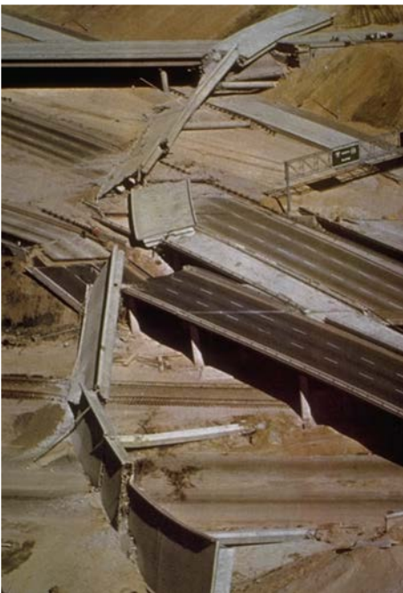
Highway Bridge Collapse – Caltrans Photo
