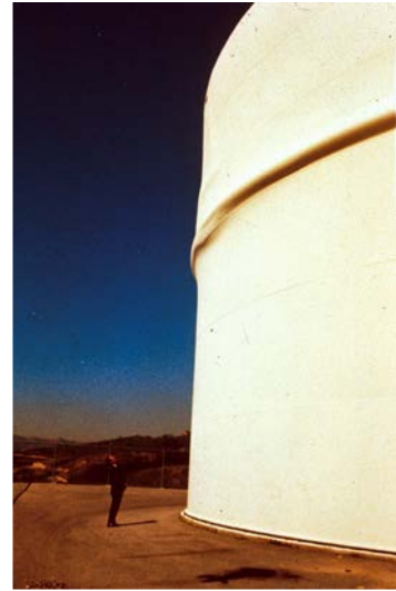
Buckle in the 2- million gallon Sesnon Tank where steel plate thickness changed from 9/16-inch to 7/16-inch – LADWP photo
