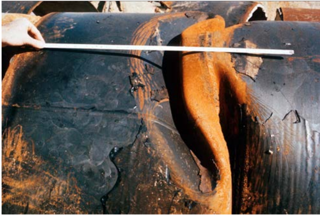
Damaged Section of the 49.5 inch diameter Granada Trunkline in the Utility Corridor – LADWP photo
