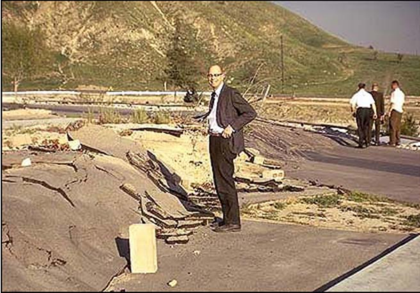
Fault rupture in Interstate 210 – Caltrans photo
