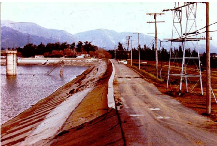
Upper San Fernando Dam showing movement of parapet wall – LADWP photo
