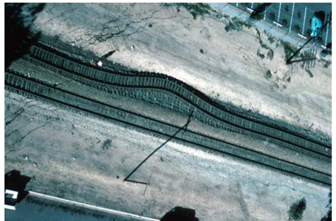
Displaced Southern Pacific Railroad tracks near Los Angeles County Juvenile Hall. – USGS Photo
