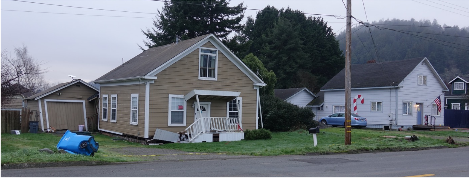
Unretrofitted - Red Tagged
